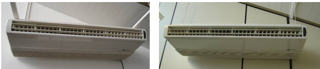
Figura 3.16 - Fan coils instalados no LabCET.
