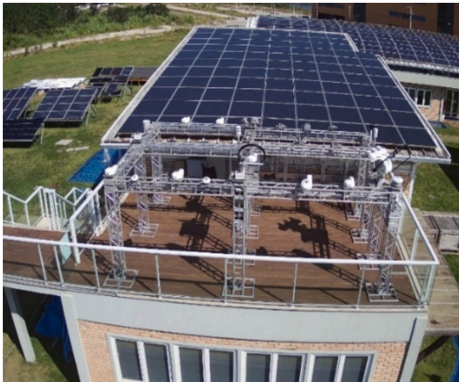
Fig. 4. The UFSC Solar Energy Research Laboratory's solar radiation measurement station in Florianópolis-Brazil.
