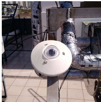
Figura 13 – Pyranometer installed on the test bed.
