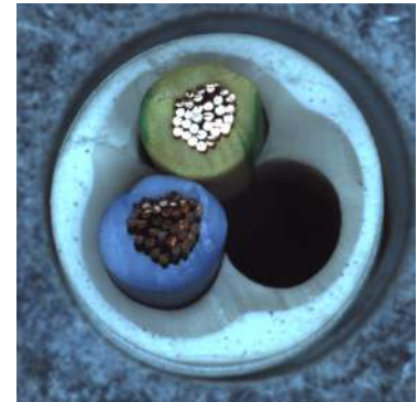
(e) Defected cable: missing cable.
