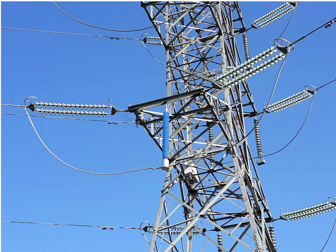
Figure 3.31 – Instrumented polymeric insulator positioned on C2 of Lages x Abdon Batista transmission line.
