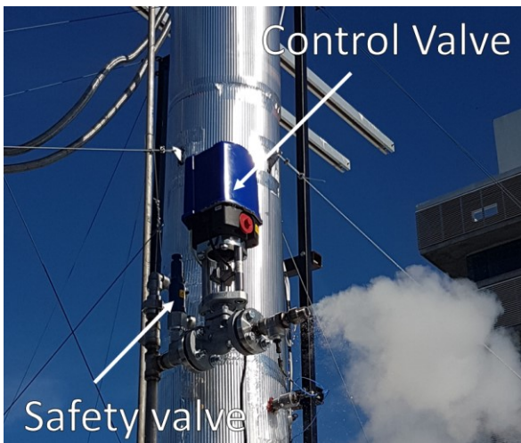
Figure B- 17 - Control and safety valves.
