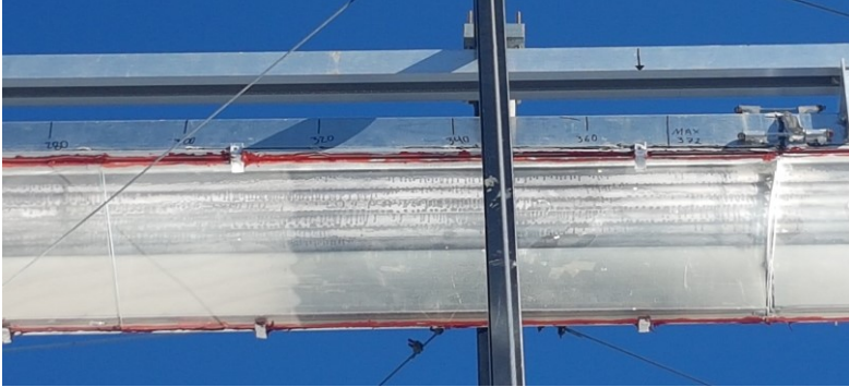
Figure D- 2 - Photo of the marked track of the moving absorber.
