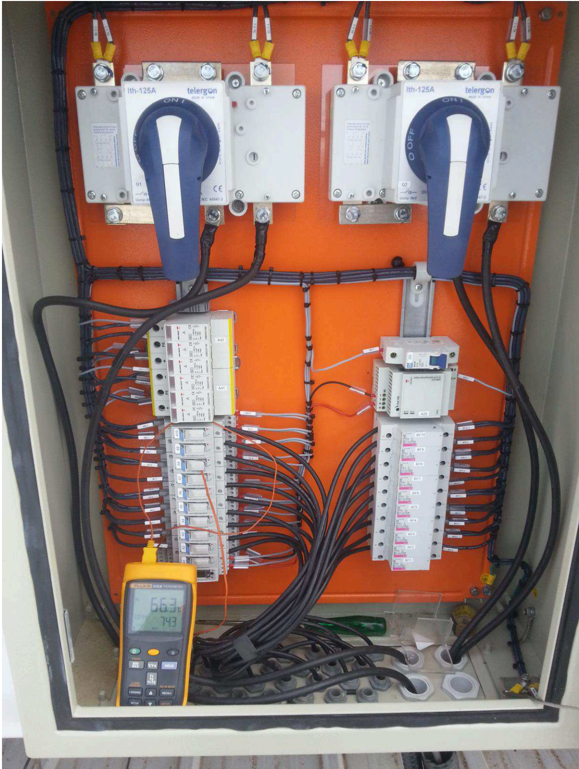
Figure 41 - Operating temperature (66.3 °C) and maximum temperature (74.3 °C) measured in a fuse holder, inside a combiner box. The meter's thermocouple is inserted in the fuse holder.
