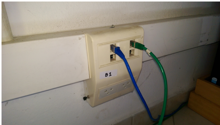
Figure 12 – Power Outlet with Smart Plug.
