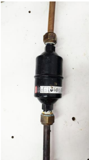
Figure 36: Picture of the filter
