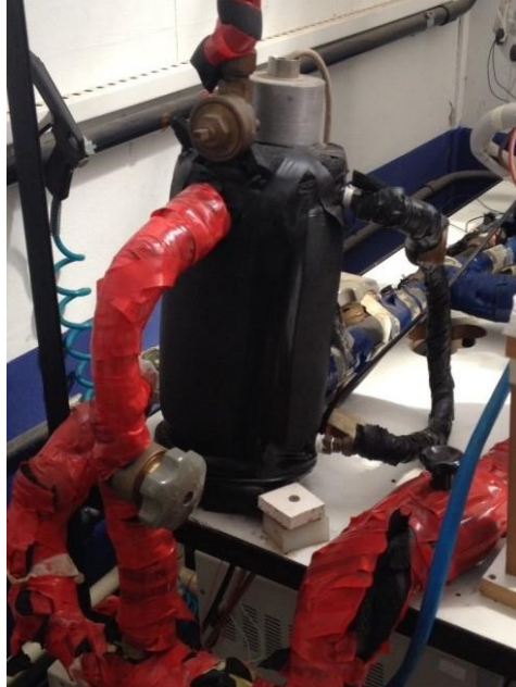
Figure B.4: Boiler at the beginning
