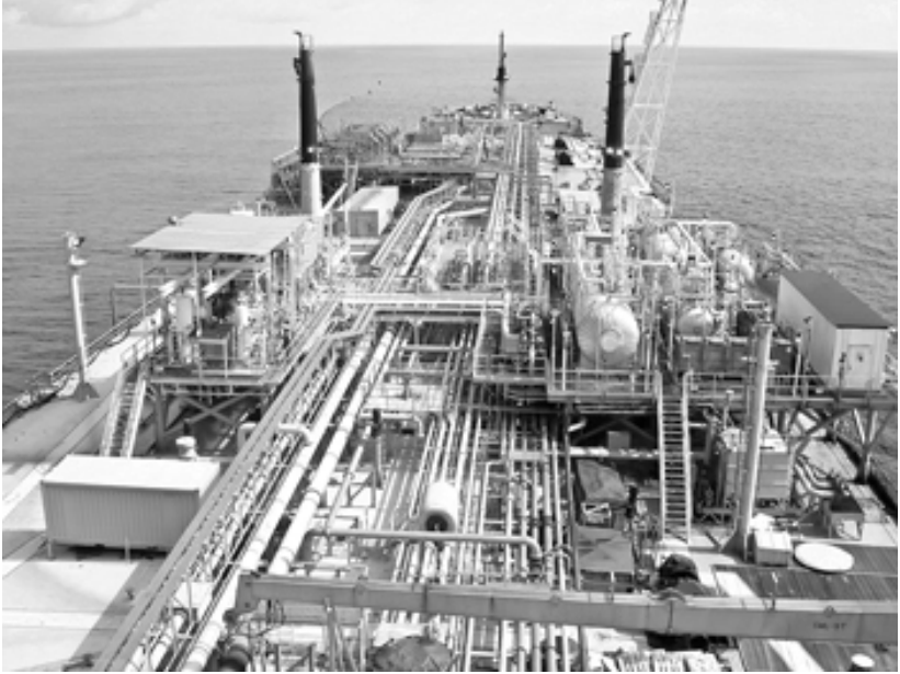
Figure 7 – Example of an FPSO topside.
