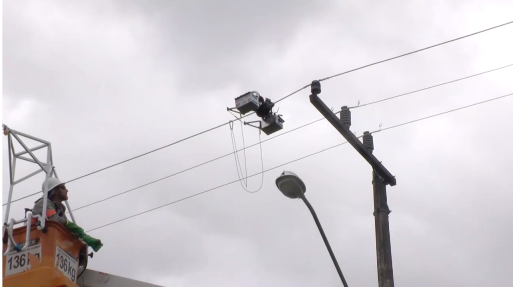
Figure 13 – Inspection robot prototype on a field test.
